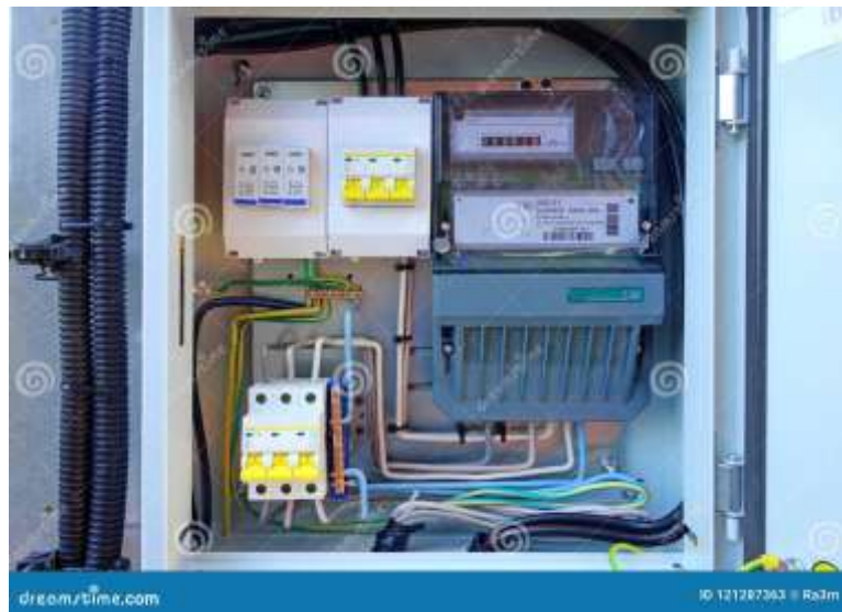
Figure 4. Three Phase Balanced three phase Meter (Dreamstime)
