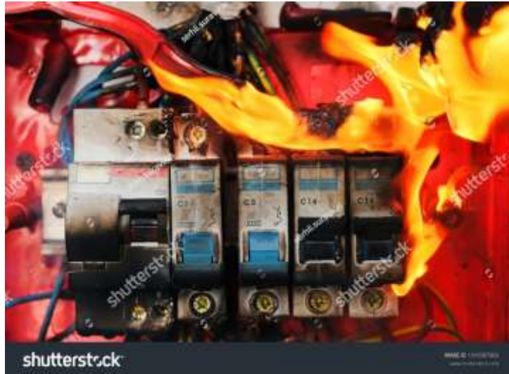
Figure 1. Burnt Electrical Breaker as a result of supply unbalance (Shutterstock)
